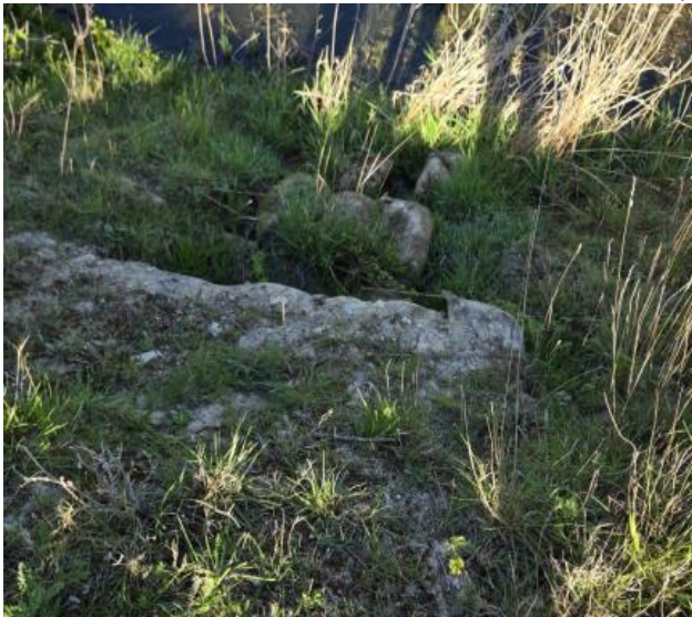
Point 20, Failing concrete bagged headwall
