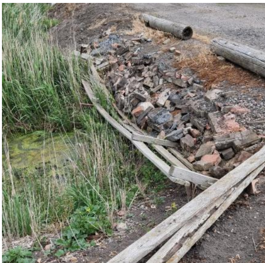
Collapsed Headwall, reach 2-11
