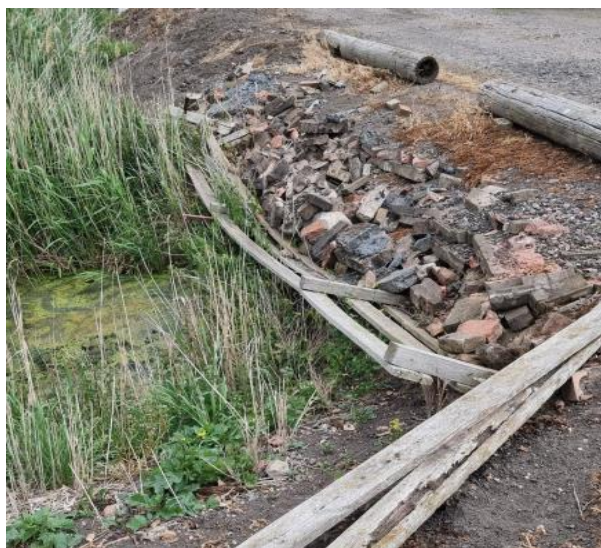
Collapsed Headwall, reach 2-11
