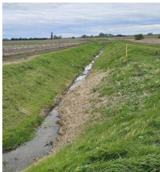
Bank Subsidence, Point 25
