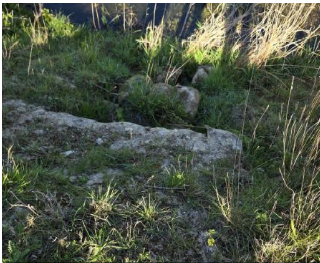
Point 20, Failing concrete bagged headwall
