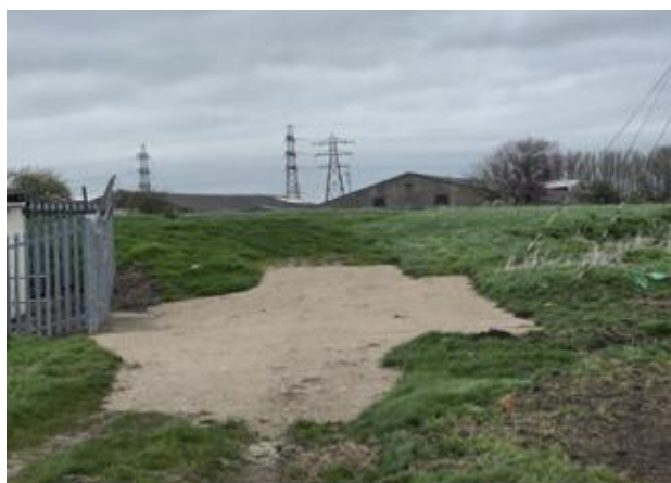
Grant funded improvements at Pumping Station to aid mobile pump deployment in the event of a breakdown
