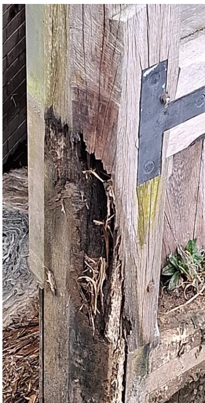
Photo showing damage to downstream doors
