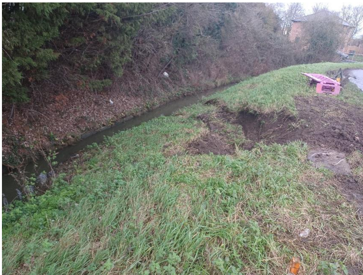
Photo showing slip at Yards End Dyke
