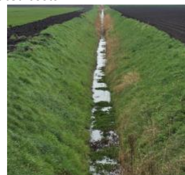
Additional Herbicide application required at point 46
