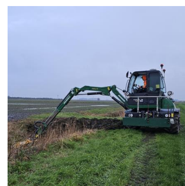
Blocked culvert, reach 83-84
