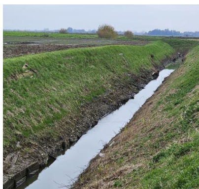
Deteriorating revetment, reach 63-64
