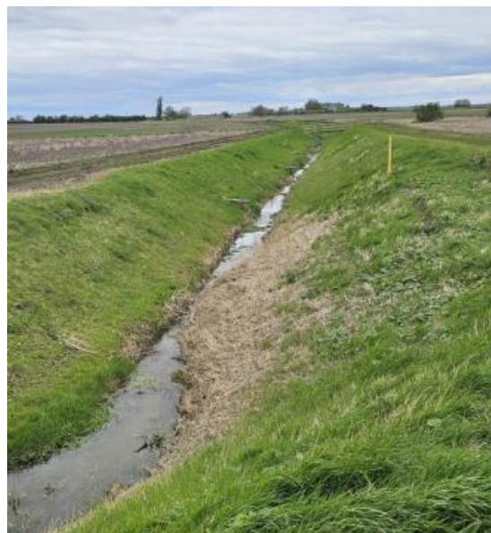
Bank Subsidence, Point 25
