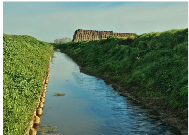
Revetment works on the left and bank subsidence on the opposite bank, reach 90-91
