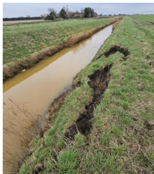
Bank Slip, downstream from Latches Fen Pumping Station, reach 40-41
