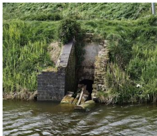
Collapsed Outlet at Point 22
