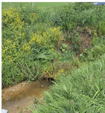
Deterioration steel culvert, Point 69
