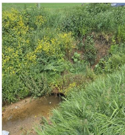
Deterioration steel culvert, Point 69
