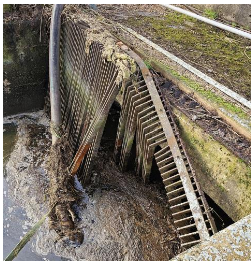
Damaged weedscreen bars and accumulations of aquatic weed
