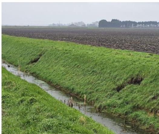
Small slips to be monitored, reach 24-25
