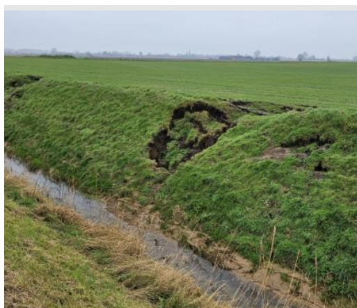
Collapsed badger setts, reach 25-26
