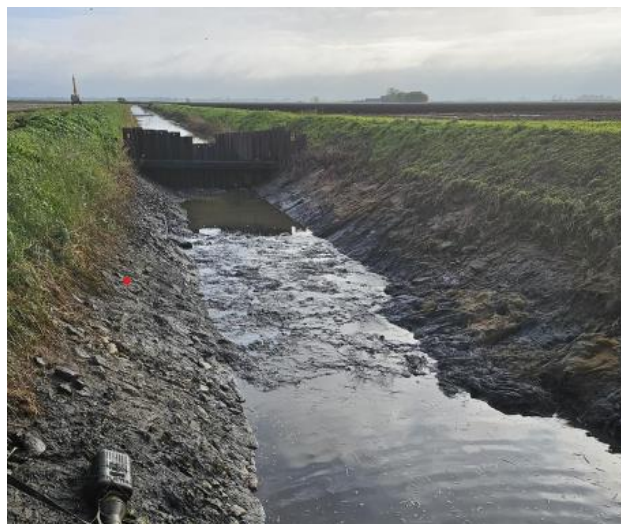
Dewatered pump drain with remnants of the weed accumulations
