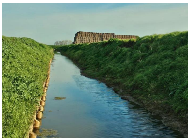
Revetment works on the left and bank subsidence on the opposite bank, reach 90-91
