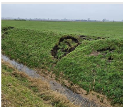
Collapsed badger setts, reach 25-26
