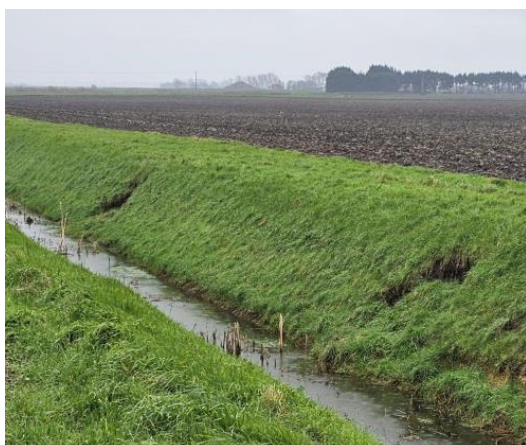
Small slips to be monitored, reach 24-25
