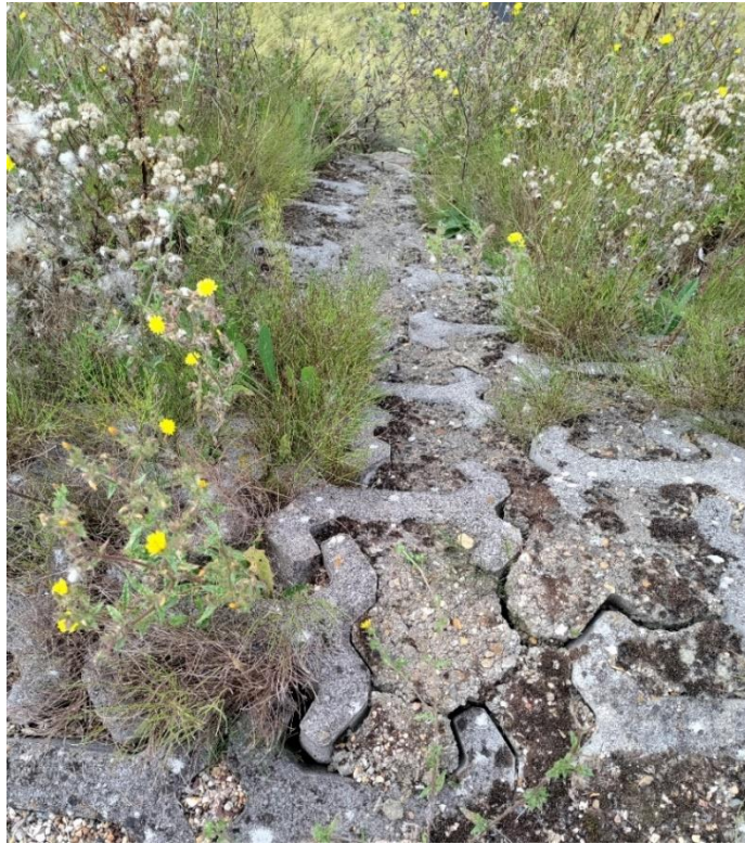
View of the cracked and deformed surface
