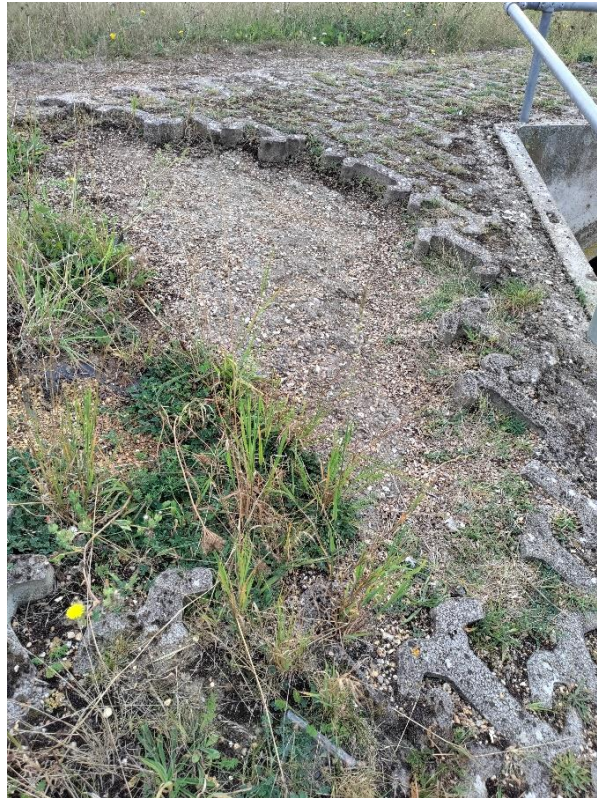
Damaged revetment at the downstream end of the surface water outfall
