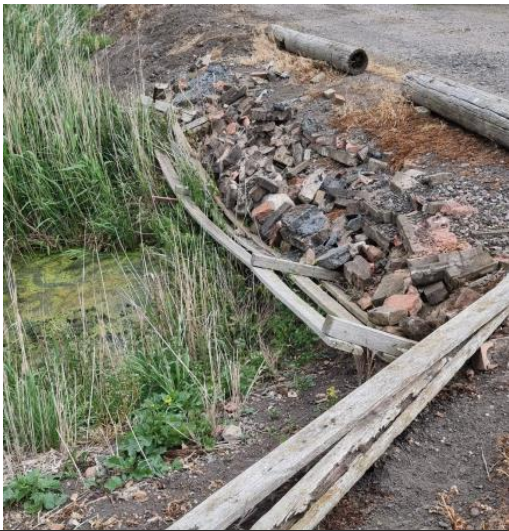
Deteriorating headwall, reach 2-11
