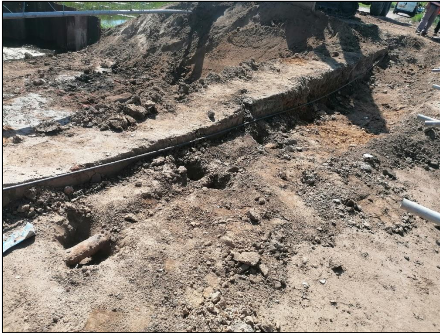
Partially Uncovered Sagging Cast Iron Water Main
