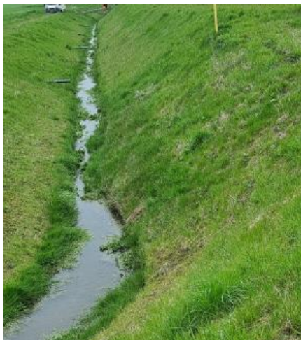
Bank subsidence, Point 25
