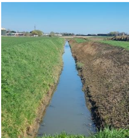
Point 33 - bank trimming on the right and the remaining steep bank on the left
