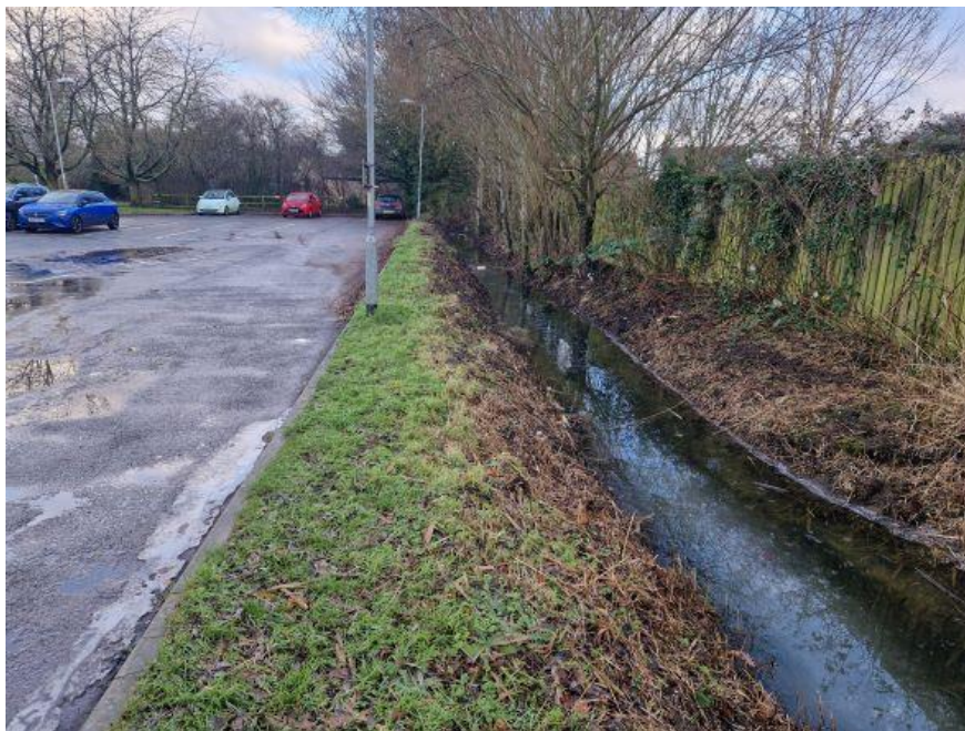
Photo showing retained water levels in ditch alongside Health Centre Carpark (26/01/23)
