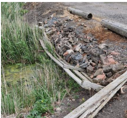
Deteriorating headwall, reach 2-11
