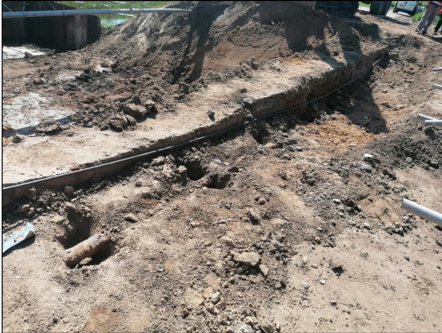
Partially Uncovered Sagging Cast Iron Water Main
