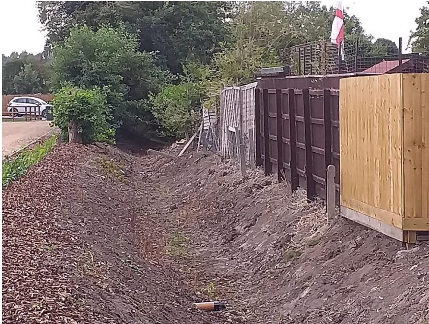
Photo showing clearance works to ditch and encroachment of opposite bank fronting Nos 36-38 Townley Close, (02/09/22)
