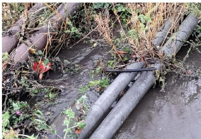
Some of the power ducts across the Sandall Road Drain between Points 58-59. The lower pipes over which the water is passing are restricting flows. Some debris is collecting.
