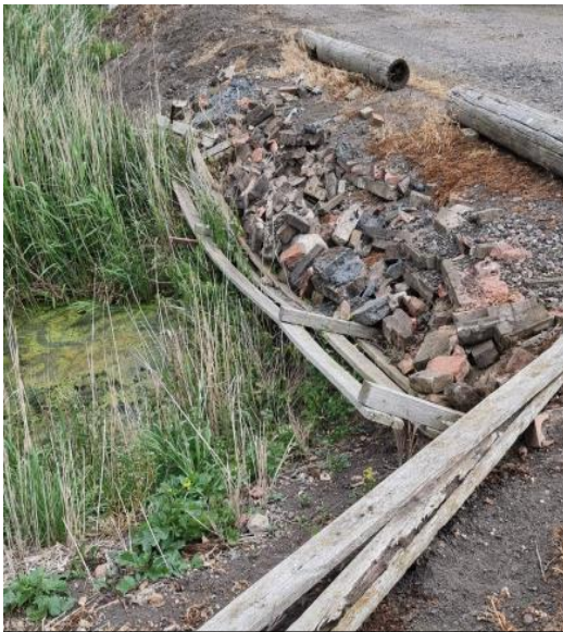
Deteriorating headwall, reach 2-11
