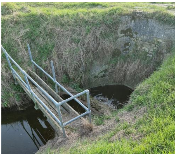
Weedscreen & Overspill, upstream of the Syphon at Point 2
