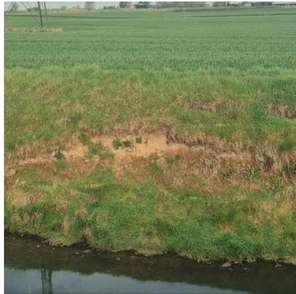
Short length of bank collapse due to steep bank profile reach 33-34
