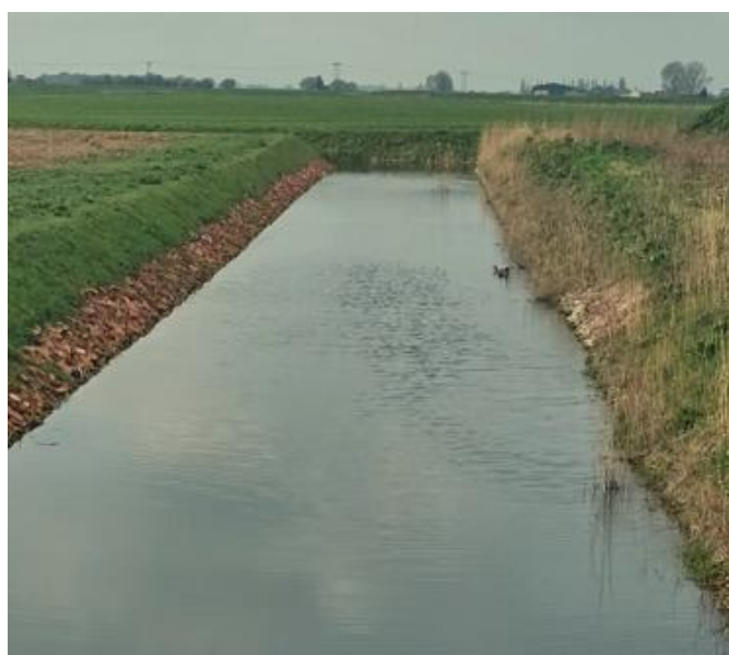
Beggars Bridge spur drain, reach 81-88
