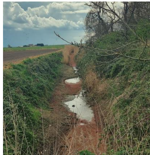
An illustration of typical bank slip occurrence, partially blocking the water channel at Point 151 exposed during low
