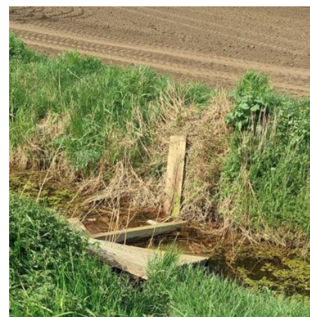
Collapsed Footbridge, reach 26-37
