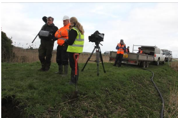
The Springwatch team spent a full day filming the construction of an otter holt.
