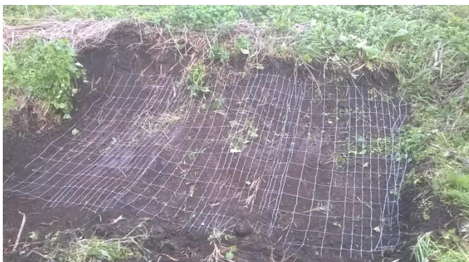
A layer of wire mesh is buried at the location of a collapsed badger tunnel to inhibit further digging at the site in the bank of New Cut near Speed the Plough.
