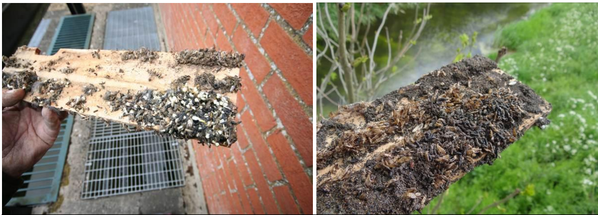
Above left, wrens droppings as well as bat droppings in a box on the Control Sluice on the Great Raveley Drain. Above right, bat droppings and earwig cases in a box beside the Forty Foot Drain near Horseway Locks.
