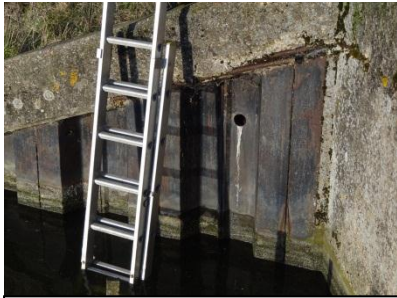
A kingfisher hole drilled on the Old River Nene near Ransonmoor Pumping Station.
