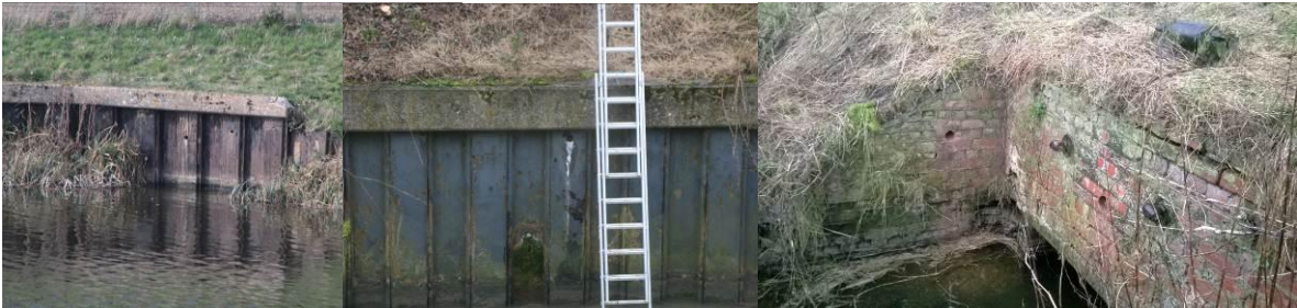
Above, left to right, potential kingfisher nesting holes drilled in piles at the former pumping station site at St Germans, at Manor Farm Bridge on the Catchwater Drain and in a culvert headwall near Pingle Bridge on the ML Main Drain.
