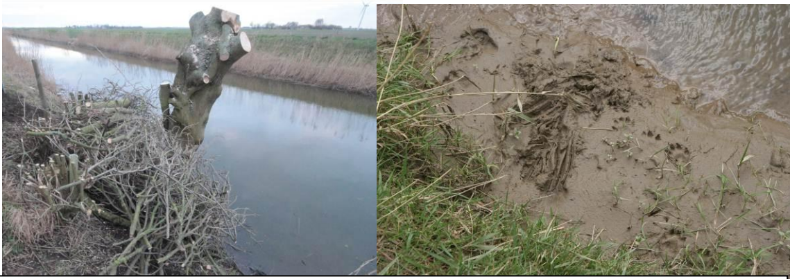
Left, a previously constructed holt at White Fen on Whittlesey Dike was refurbished and expanded using wood from pollarding the adjacent ash tree. Visitors to the original holt recorded in a single night on a trail camera included weasel, mink, rabbit, rat and bank vole. Right, otter spraints and prints were present at many of the Hundred Foot Washes IDB inlets in April.
