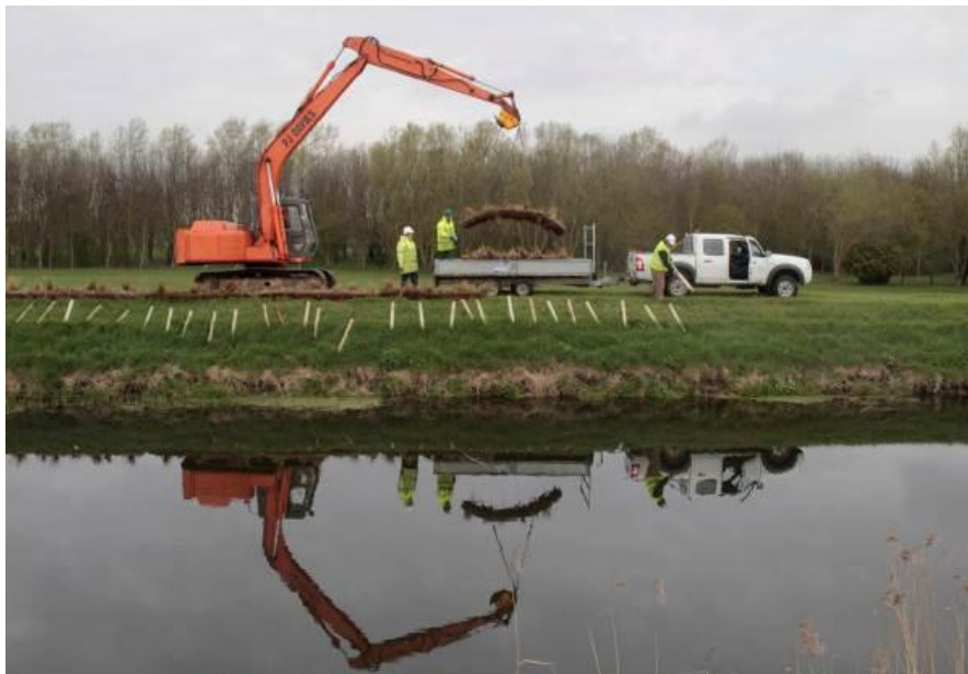
Coir rolls being prepared for installation on the margin of the Old River Nene near Lodes End Locks.
