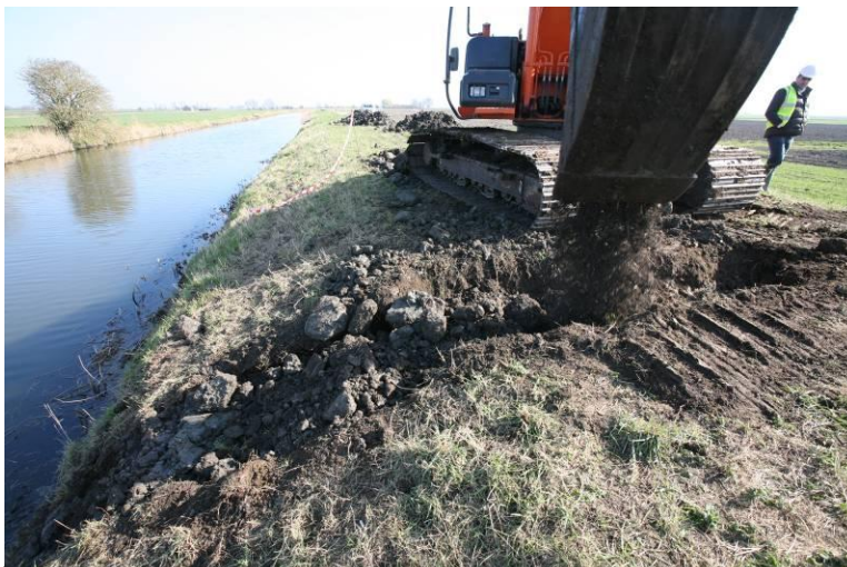
The badger tunnel being filled with clay on the side of the Black Ham.
