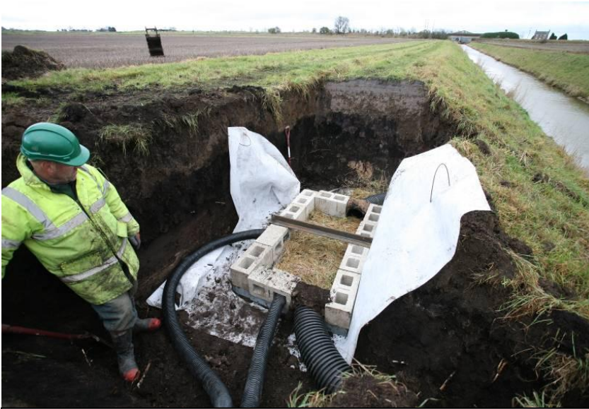
An otter holt in the process of construction alongside a Curf & Wimblington Combined IDB drain.
